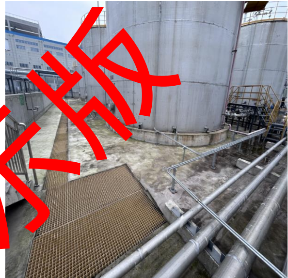
NMP 罐区围堰、截流沟及收集井
